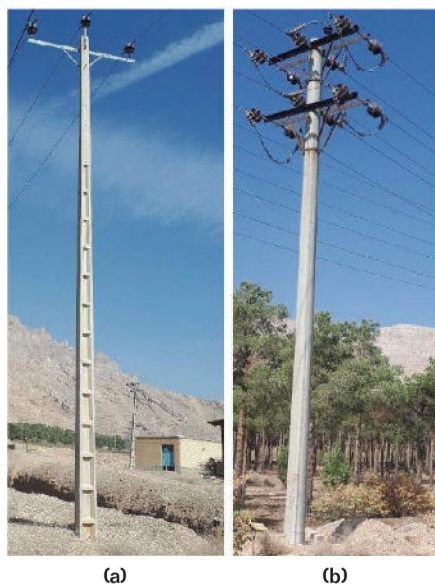
FIGURE 1 Two different types of concrete poles: (a) H cross section, and (b) round cross section or O section.
