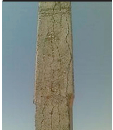
The concrete cover on this power pole cracked and fell off as a result of high-voltage AC leakage.
