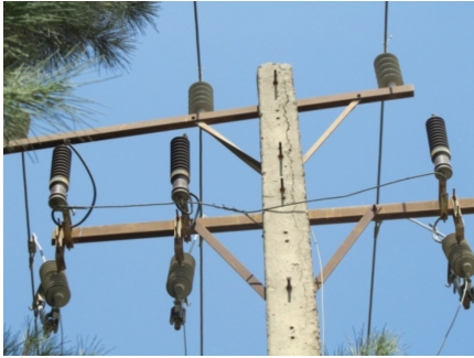
FIGURE 2 A rusty galvanized cross arm in the polluted atmosphere of Dolatabad.
