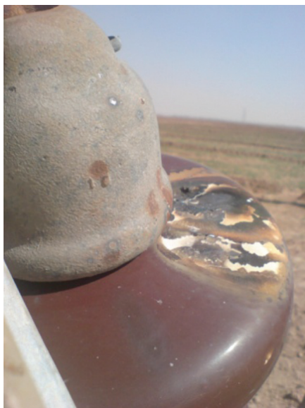
FIGURE 5 Typical punching of the surface of an insulator after experiencing creep current.
