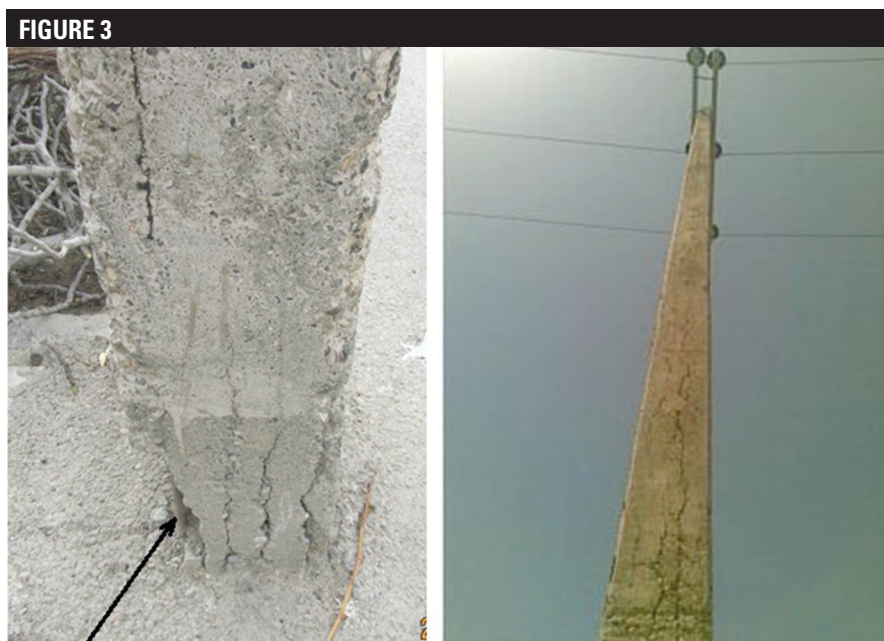
Rebar without visual corrosion Cracks in concrete power pole caused by stray AC.
